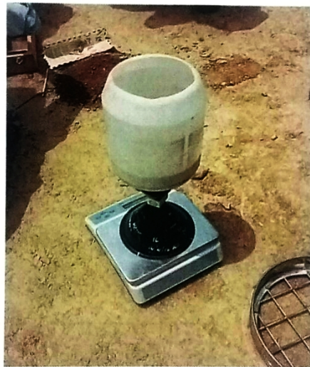
Figure No. 4.2 sand cone apparatus (image taken from field test on motoway )
