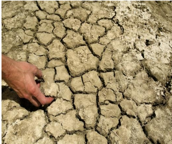
Figure 1.1 Cracks in clayey soils due to shrink-swell behavior.
