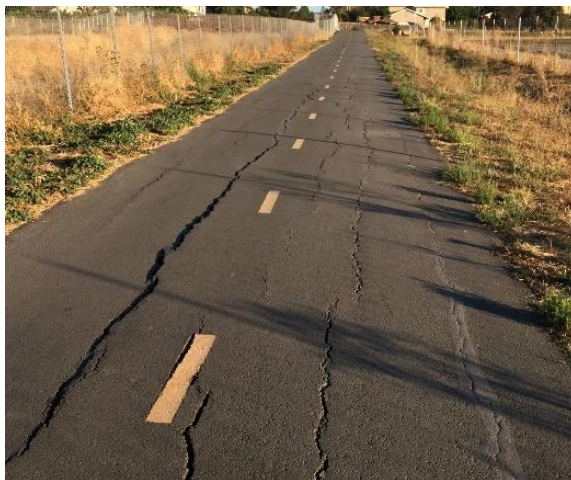
Figure 1.2 Road failure due to low strength subgrade soil.
